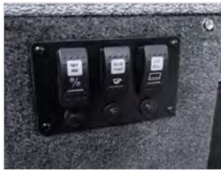
Illuminated switches are visible and always within reach.
